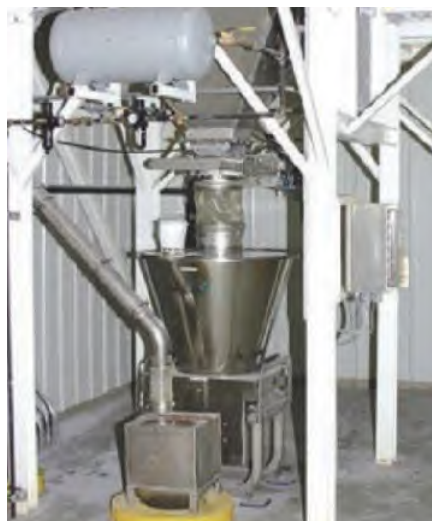
Stainless Steel loss-in-weight product delivery system feeding our granulation equipment
