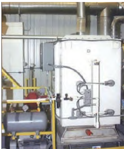
Cartridge filter baghouse with metered air flow to optimize efficiency
