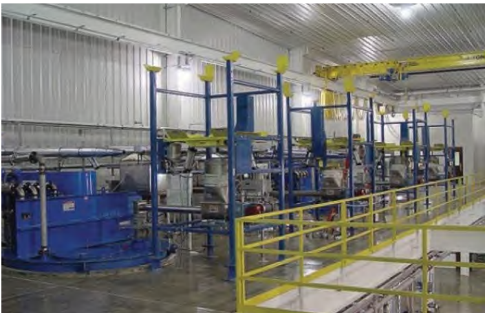
Solid Batching Stations
